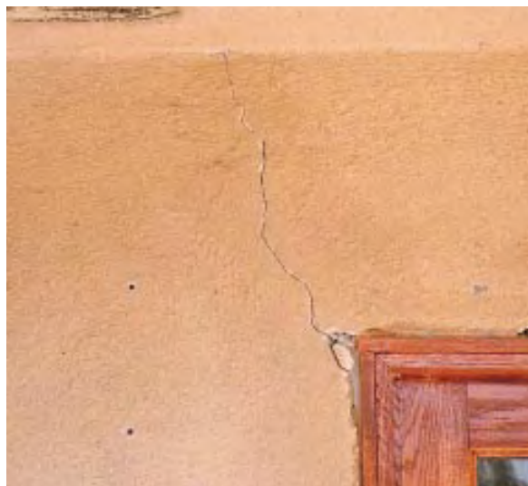
Figure 14. Stucco cracking is one of the most common customer complaints. Tight surface cracks are normal in stucco and can usually be repaired. With quality workmanship, larger cracks can be avoided.
