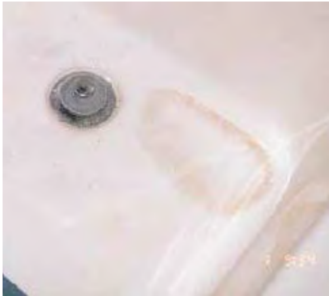
Figure 19. Ponding in the bottom of a tub unit — the result of an out-of-level installation — is not structurally serious but is obvious to any homeowner.
