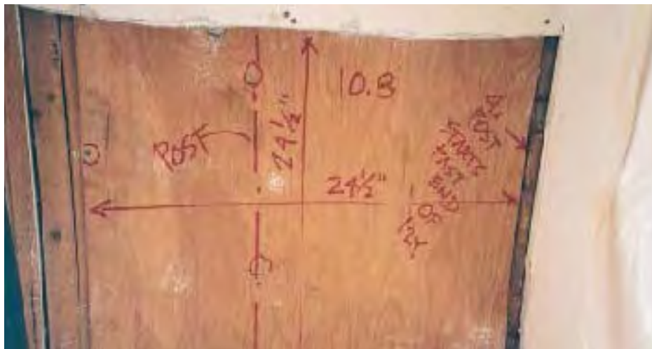
Figure 3. This shear plywood falls short of the shear wall posts on the right and left, and is attached with too few nails.
