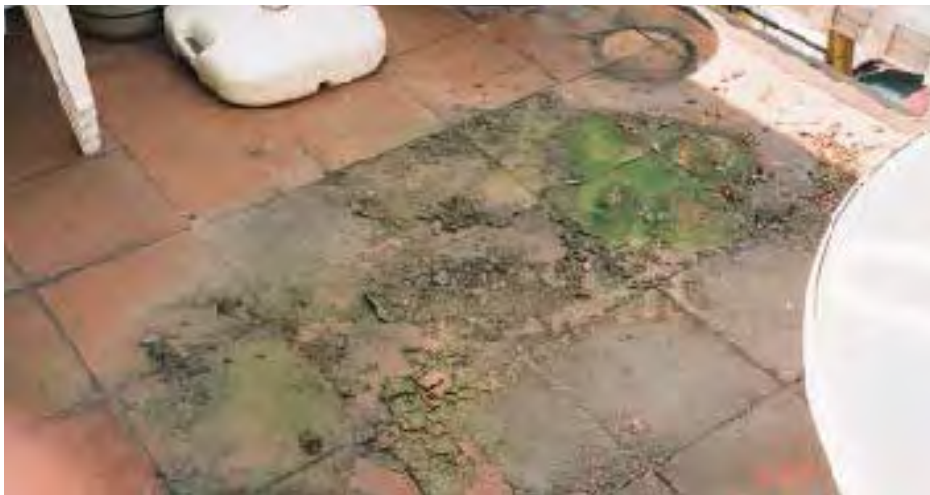
Figure 16. Besides ruining the finish surface, ponding on waterproof decks also leads to deterioration of the framing below.
