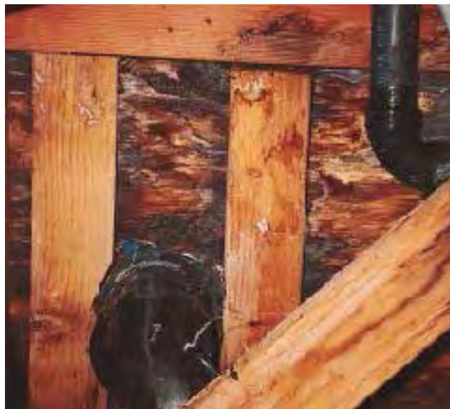
Figure 17. If hidden by finish surfaces, a leaky toilet connection can go undetected until structural decay sets in.
