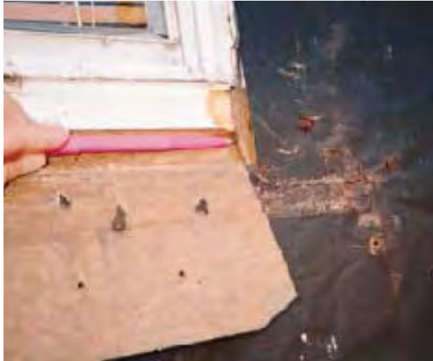
Figure 10. Here, the building paper is installed under the flashing paper at the bottom of the window, but not on the side — leaving a vulnerable corner where the flashing paper has been cut.
