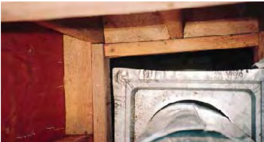
Figure 22. Firestops are an important safety requirement. Unfortunately, if a gap is missed by the inspector, all too often it will be permanently concealed from view.
