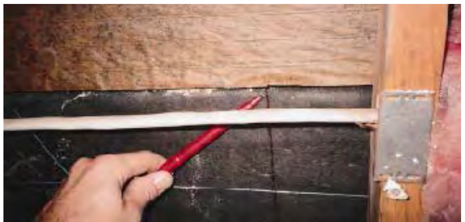
Figure 9. The building paper below a window must be tucked below the flashing paper — a detail often botched, as in the top photo. Above is a reverse lap seen from the inside of the wall cavity.
