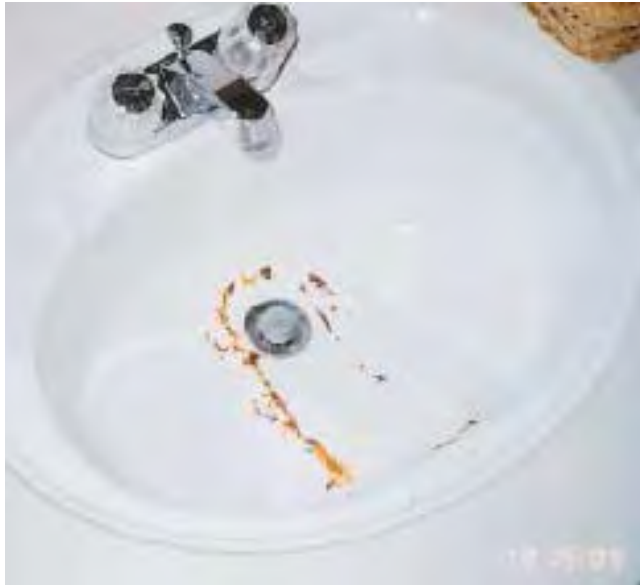
Figure 18. The chipped enamel in this cheap lavatory sink is the kind of defect that will send condo or tract homeowners ballistic — especially when they see it in every home on the block.
