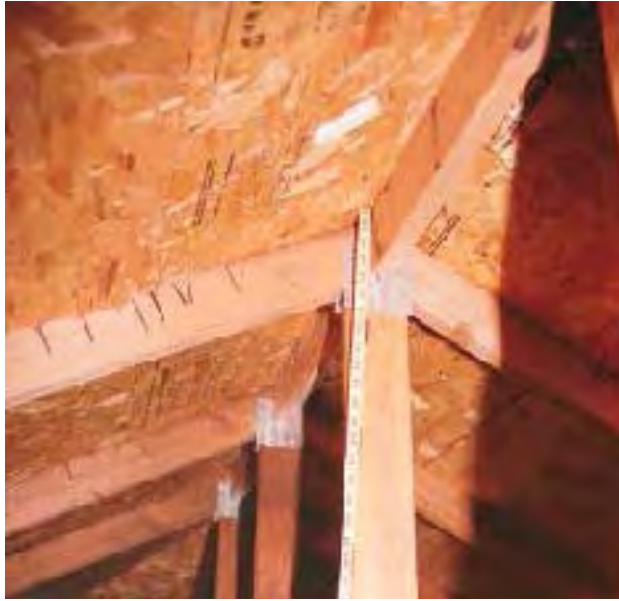
Figure 1. Nails that miss the truss — a result of sloppy work with a pneumatic nailer — void the strength of the roof diaphragm.
