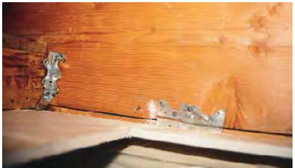
Figure 6. An inspection made through a hole cut in the ceiling reveals that the joist hanger at left is bent and missing nails.
