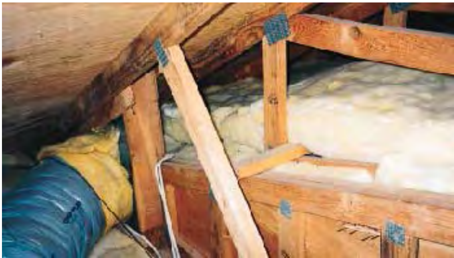
Figure 2. The plywood on this interior shear wall should have been carried all the way to the roof diaphragm.
