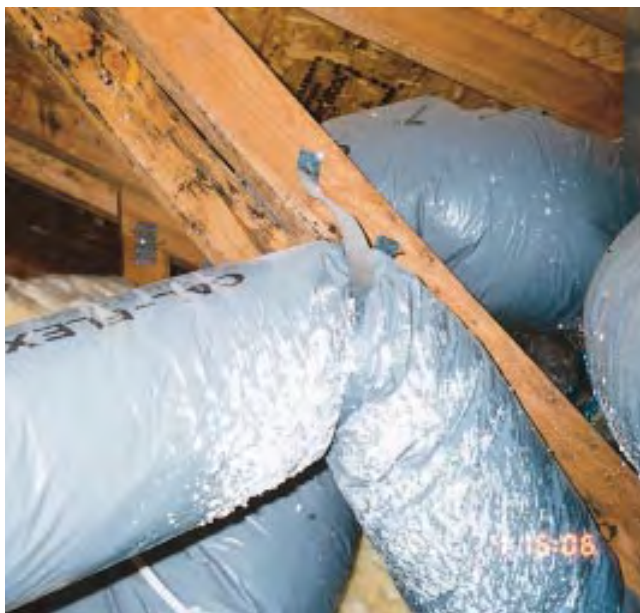
Figure 20. A pinched duct can result in uneven temperatures. It's easy to fix if it's accessible, but easier still to avoid.
