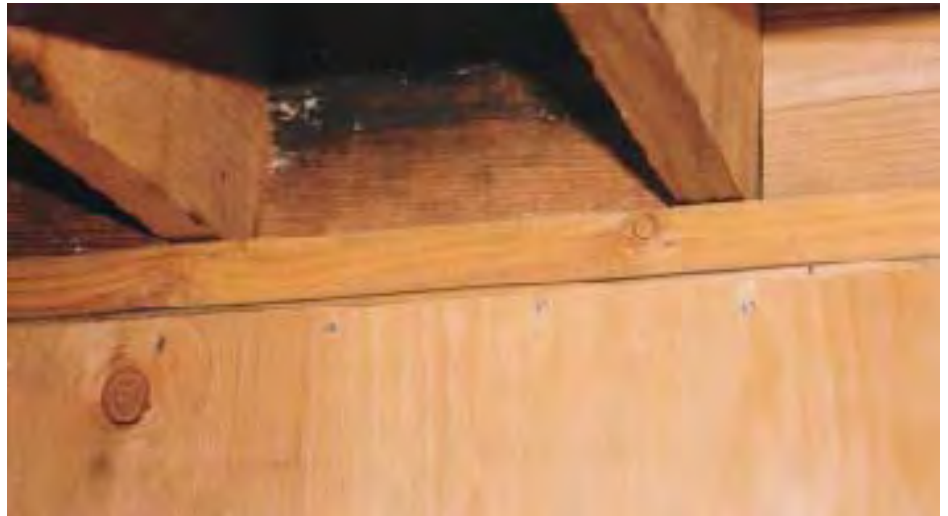
Figure 4. This shear plywood should have extended to the top of the double top plate — a mistake that can be remedied with the addition of metal connectors across the two plates.
