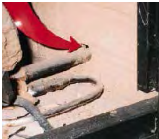
Figure 23. The pipe penetration into a gas fireplace must be properly sealed with a firestop material — a defect that's easy to spot and easy to fix with fireproof grout.
